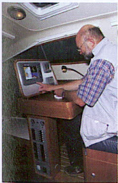
ABOVE: The navigation area has a large instrument console, and Northshore is offering two seats at the chart table as an option
